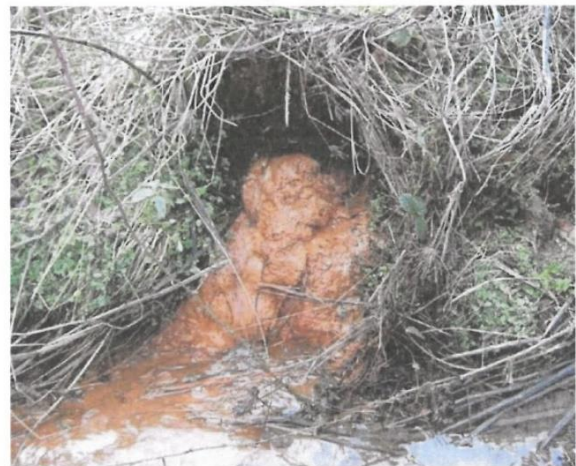
Figure 24. Drainage outfall blocked by ochre
