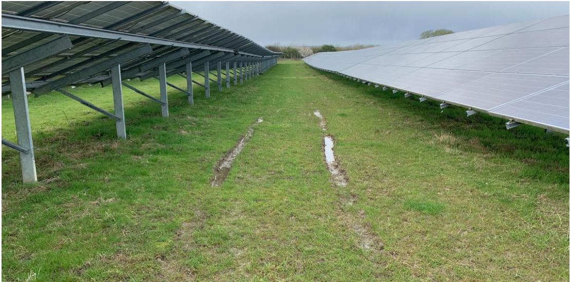
Photo 31: Ruts Caused by Vehicles
