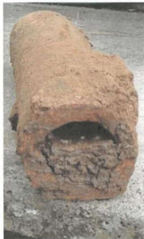
Figure 22. Silted clay drain
