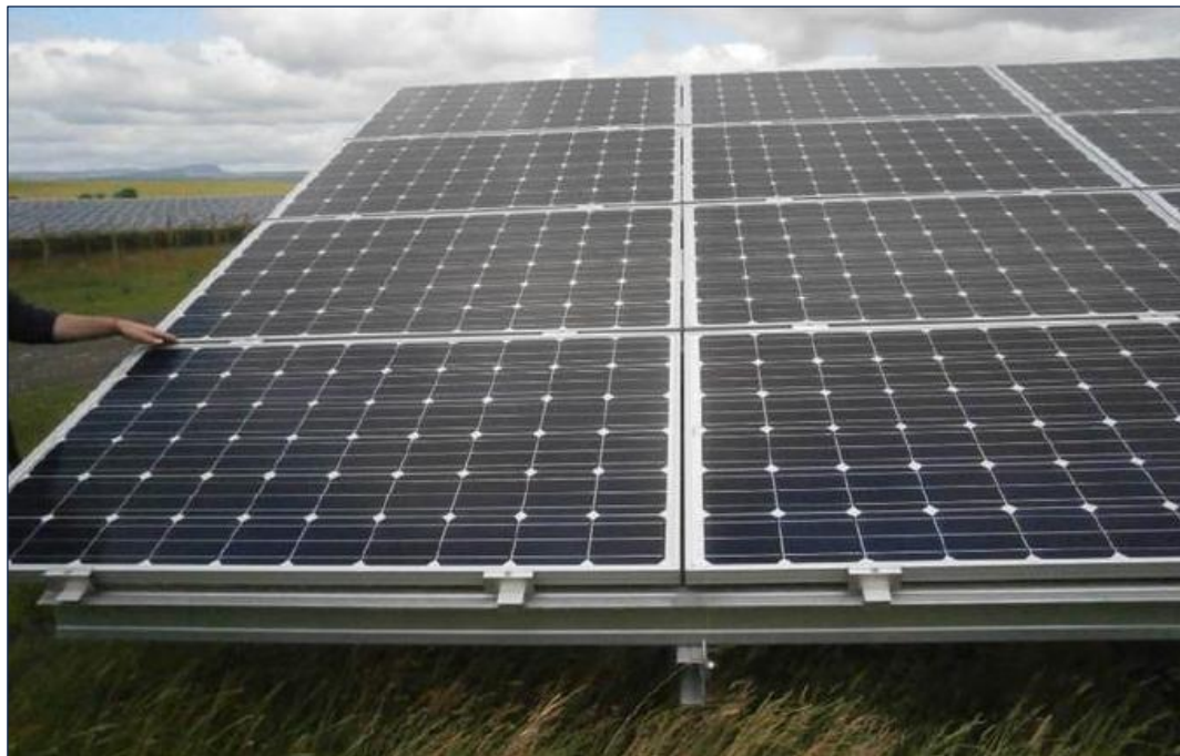
Figure 6-1 Typical Solar Panel Arrangement (showing expansion gaps)
